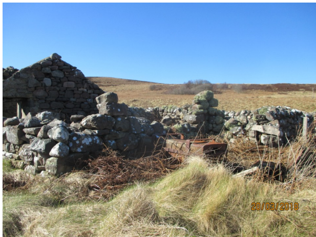
The building has been altered but the construction is of dressed stone that is layered with lime mortar used in the walls and a cement cap on the skewes.
